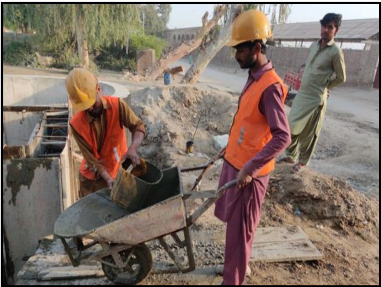
WW-09 (Zone-C) Concrete pouring of Screen Chamber work is in progress at Railway Station Jacobabad
