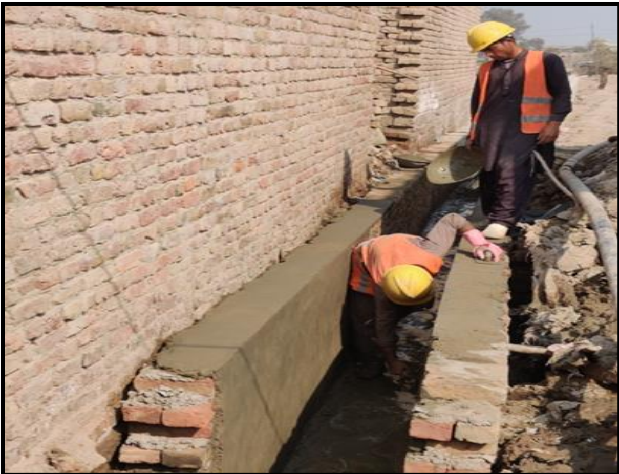
WW-08 (Zone-B) Plaster and brick masonry of drain work is in progress at street No. 13D Al Murtaza Colony Jacobabad
