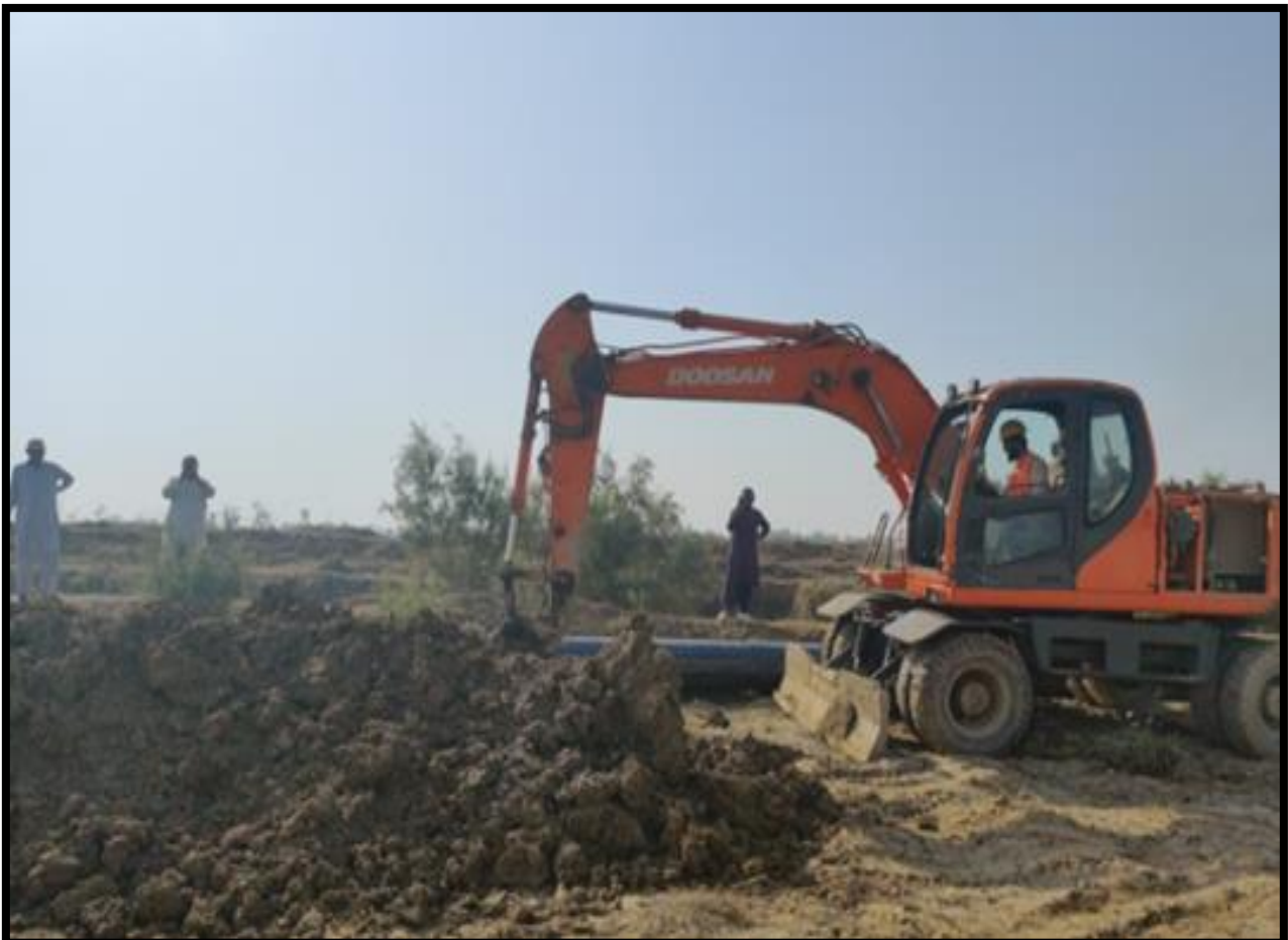
WW-12 (Zone-C) Excavation for 500mm dia pipe for Rising main work is in progress at Shamb-e-Shah to Noorwah Jacobabad
