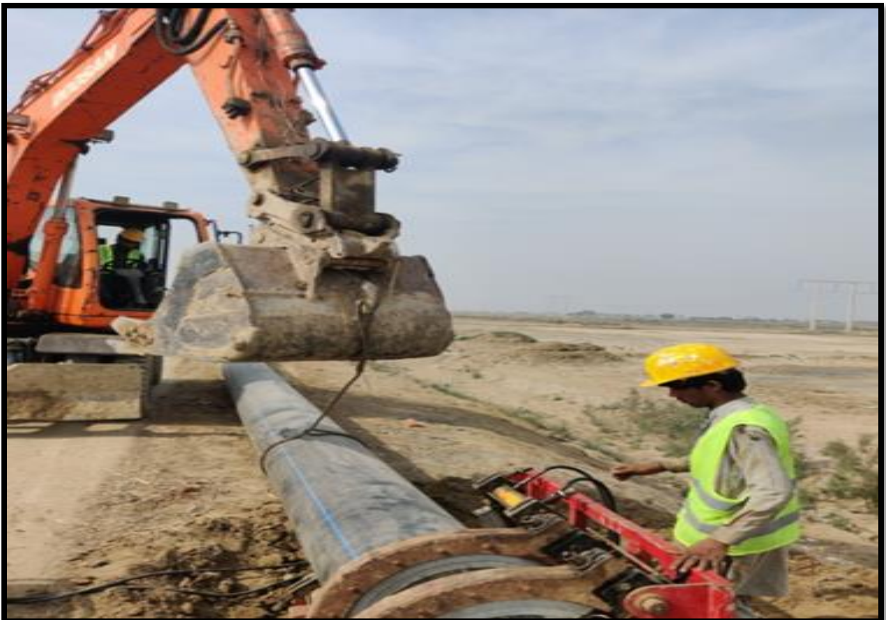
WW-12 (Zone-C) Jointing of the 500mm dia pipe for Rising main work is in progress at Shamb-e-Shah to Noorwah Jacobabad
