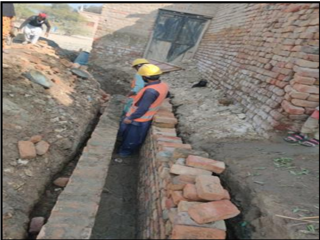
WW-08 (Zone-B) Brick masonry of drain work is in progress at street No. 13-F Al Murtaza Colony Jacobabad
