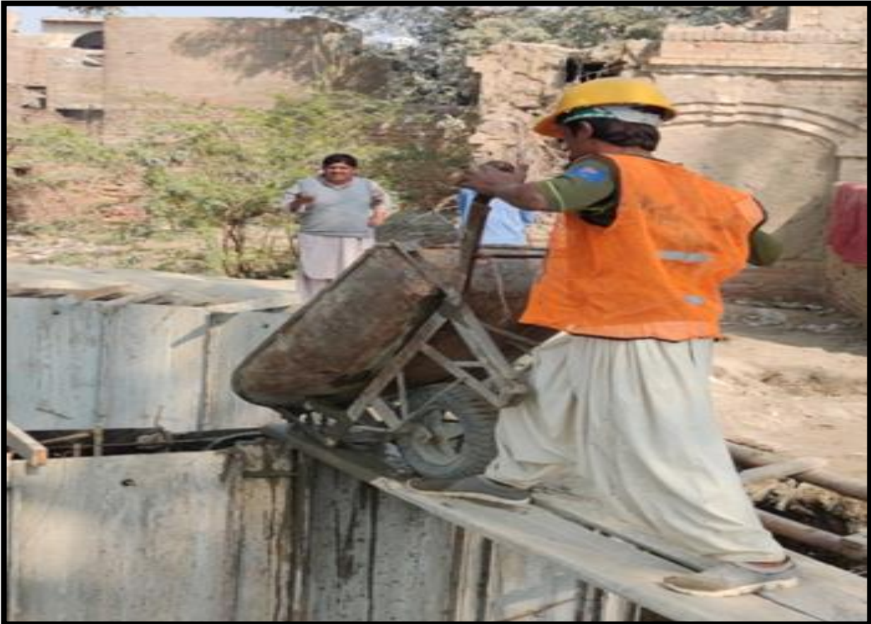
WW-09 (Zone-C) Concrete pouring of sump wall work is in progress Railway Station Jacobabad
