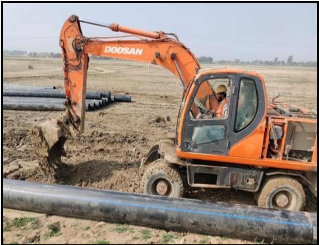
WW-12 (Zone-C) Excavation for 500mm dia pipe for Rising main work is in progress at Shamb-e-Shah to Noorwah Jacobabad
