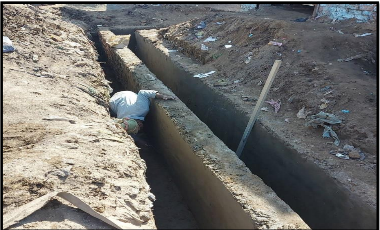
WW-08 (Zone-B) Plaster of Brick masonry of drain type 3 work in progress at Al Murtaza Colony Jacobabad
