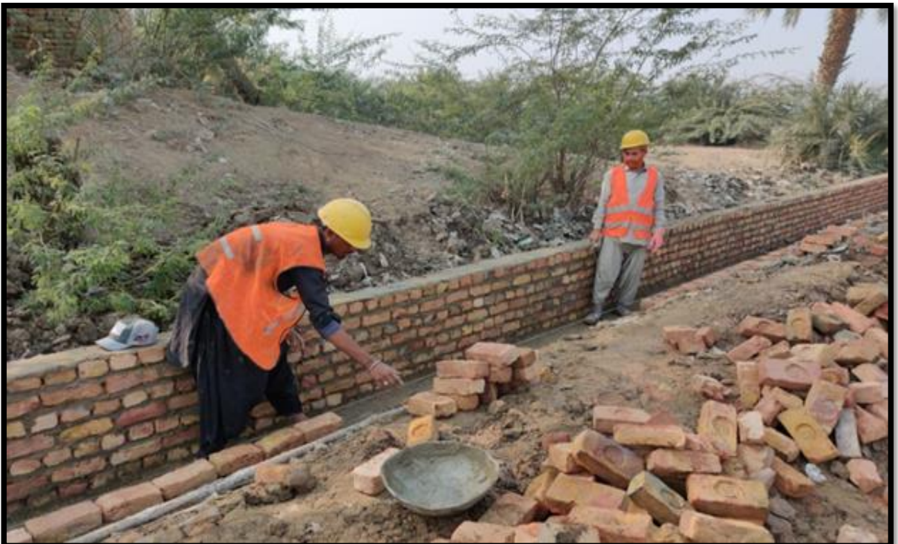
WW-08 (Zone-B) Brick masonry of drain work in progress at street No. 11-B, Al Murtaza Colony Jacobabad
