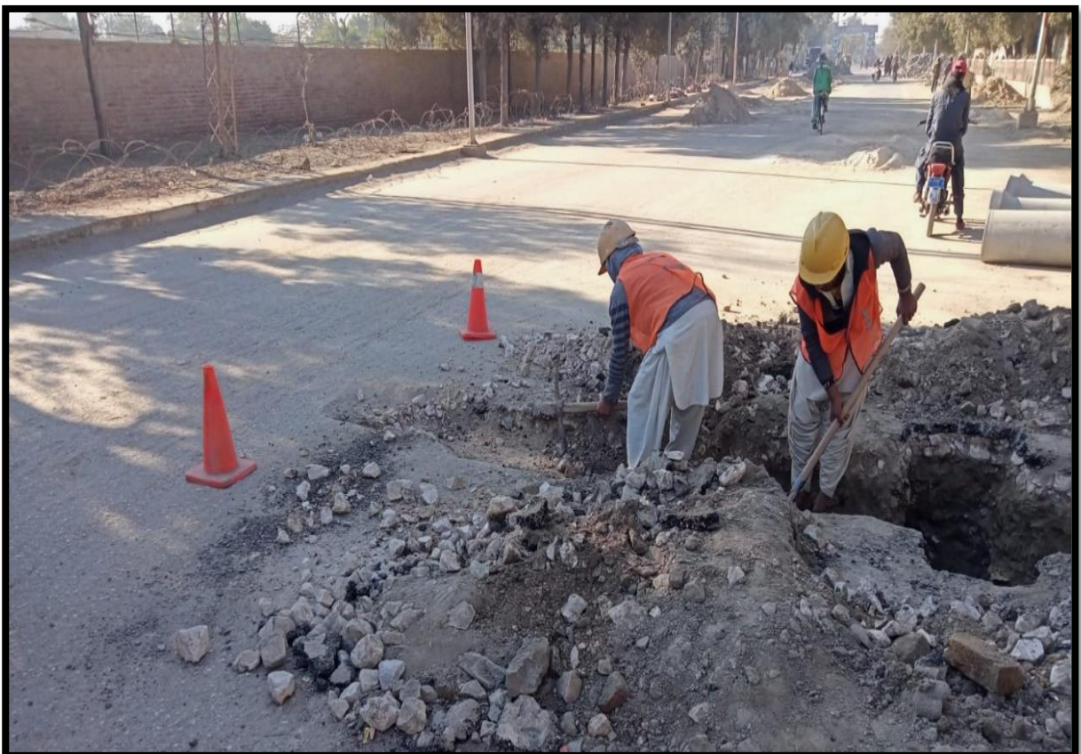
WW-07 (Zone-A) RCC Casing work for Raising Main work in progress at Revenue Colony Jacobabad
