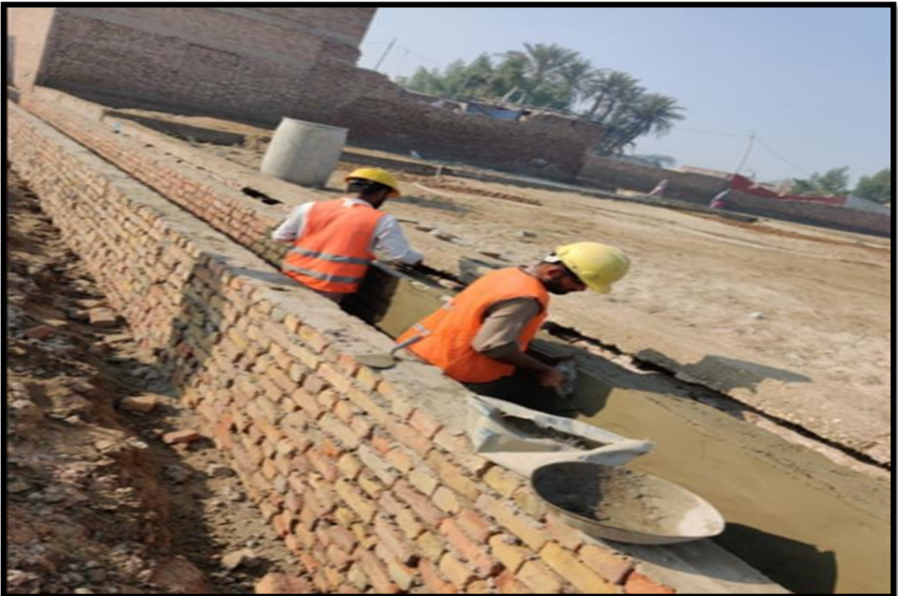
WW-08 (Zone-B) Plaster of brick masonry work in progress at street No. 11-A Al Murtaza Colony Jacobabad
