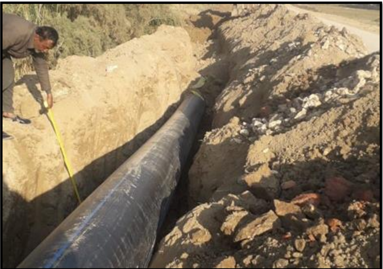
WW-12 (Zone-C) Raising Main 500 mm diameter PE Pipeline work in progress at Hambi road Jacobabad
