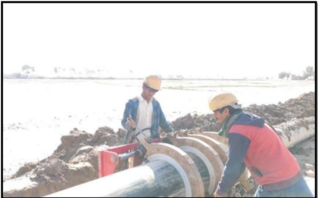
WW-12 (Zone-C) Jointing of HDPE500 mm diameter Pipe for Raising Main work is in progress at Shamb-e-Shah to Noor Wah Jacobabad
