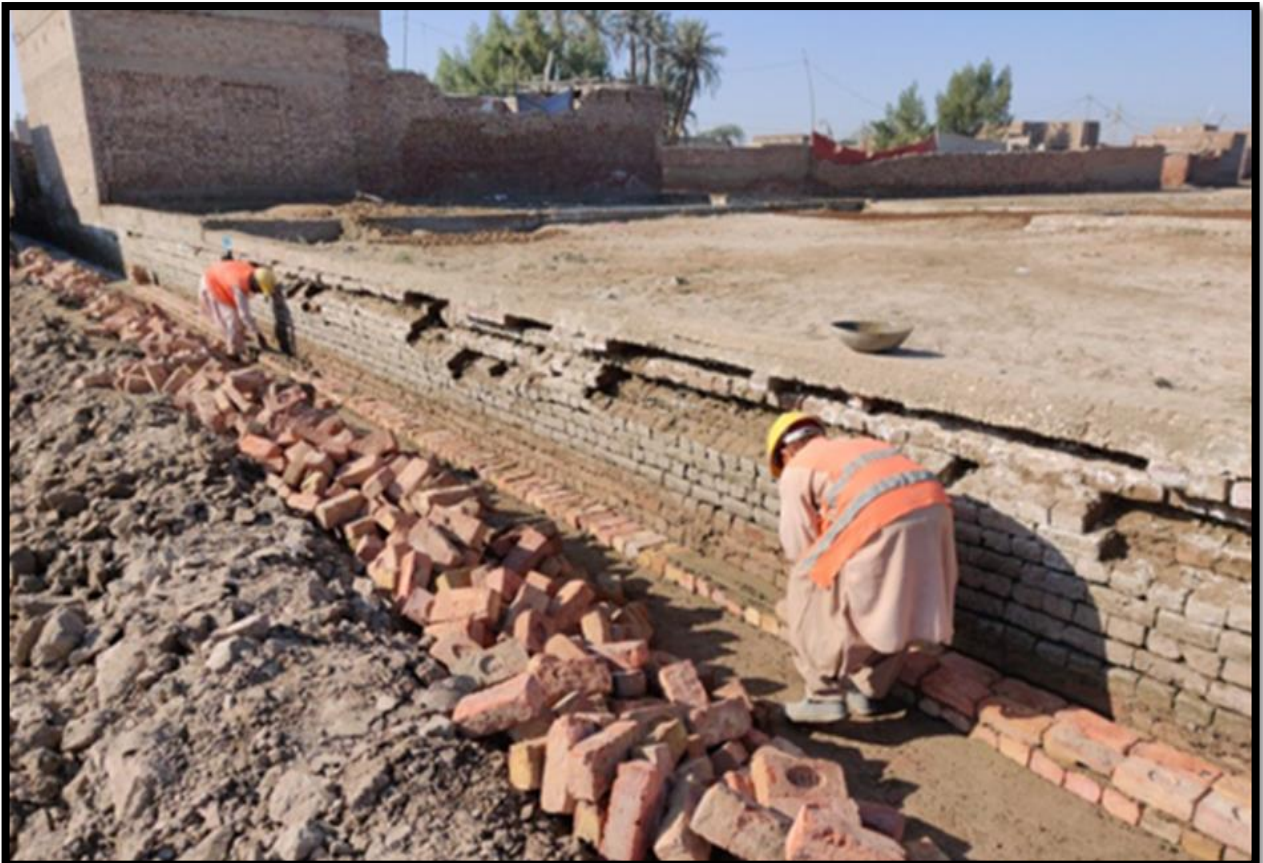
WW-08 (Zone-B) Plaster of brick masonry work in progress at street No. 13-D Al Murtaza Colony Jacobabad
