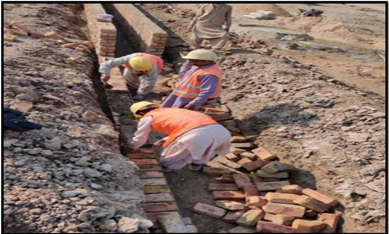
WW-08 (Zone-B) Brick Masonry of drain work in progress at Street No. 13-D, Al Murtaza Colony Jacobabad
