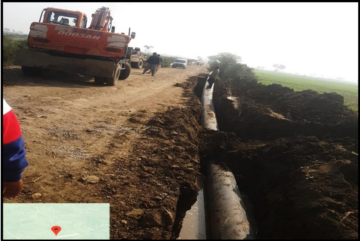
WW-12 Rising main 500 dia work is in progress from Shamb-e-Shah to Noor Wah Jacobabad
