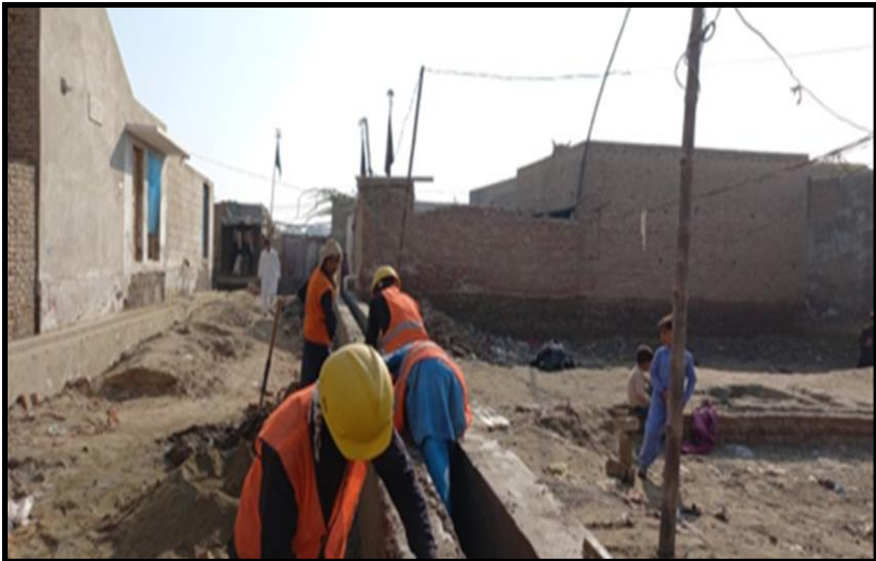
WW-08 (Zone-B) Brick Masonry work of drain is in progress at street No 2-C Al Murtaza Colony Jacobabad
