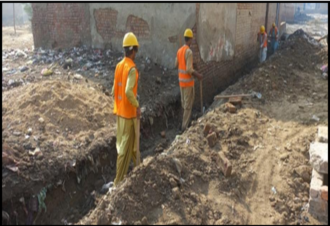
WW-08 (Zone-B) Excavation of drain work is in progress at street No. 7-C Al Murtaza Colony Jacobabad
