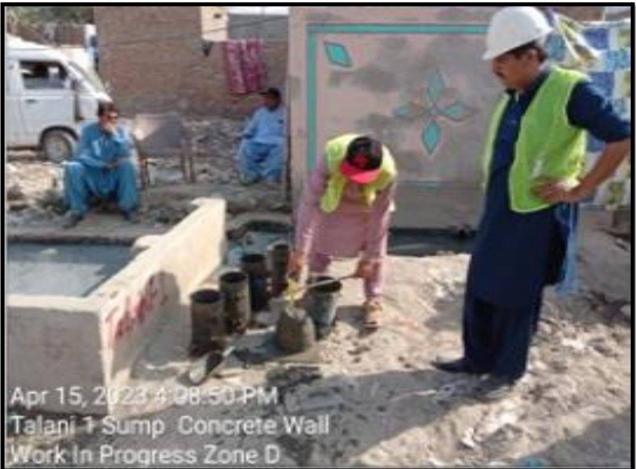
WW-10 (Zone-D) Sump Cone & Cylinder process of concrete pouring of Sump Talani-I work in progress
