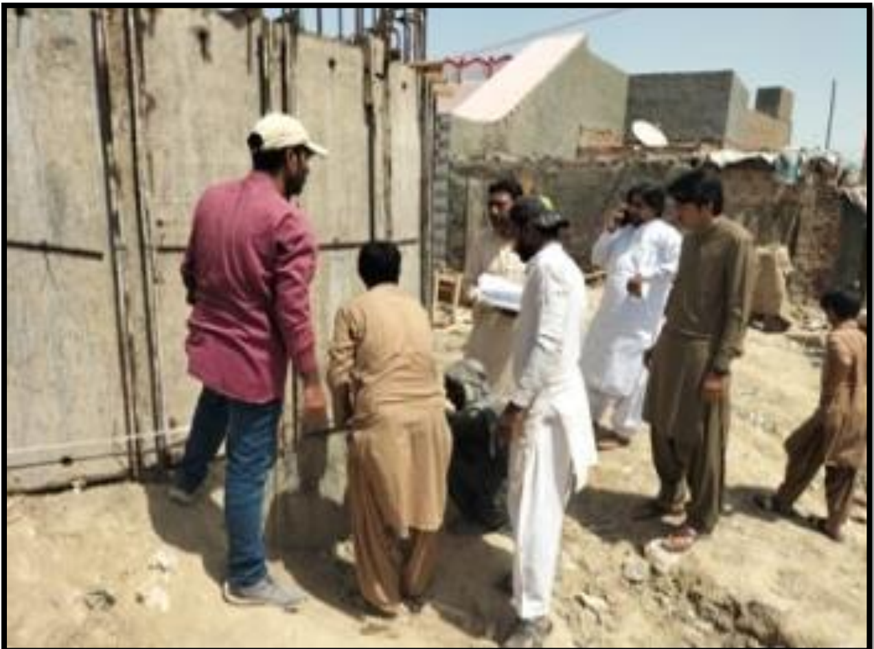
WW-07 (Zone-A) Check/monitor the dimension of Sump at ADC Colony work in progress
