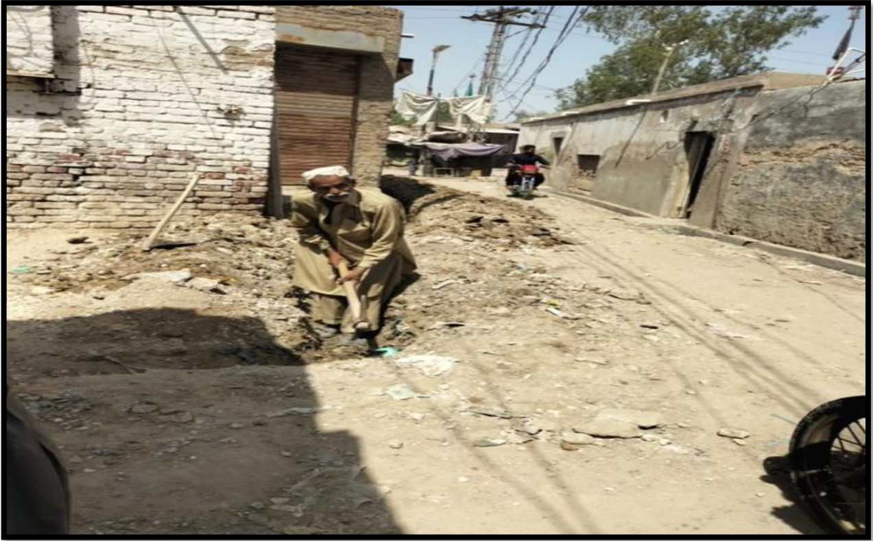
WW-07 (Zone-A) Excavation for temporary diversion for Railway colony Sump work in progress
