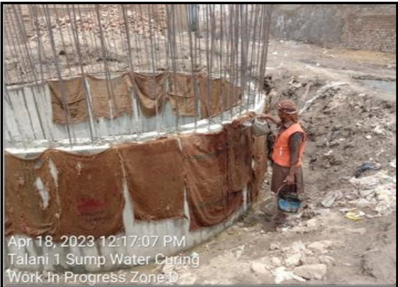
(Zone D) Bitumen Coating of Pachua Sump & Water curing of Talani-I Sump work in progress
