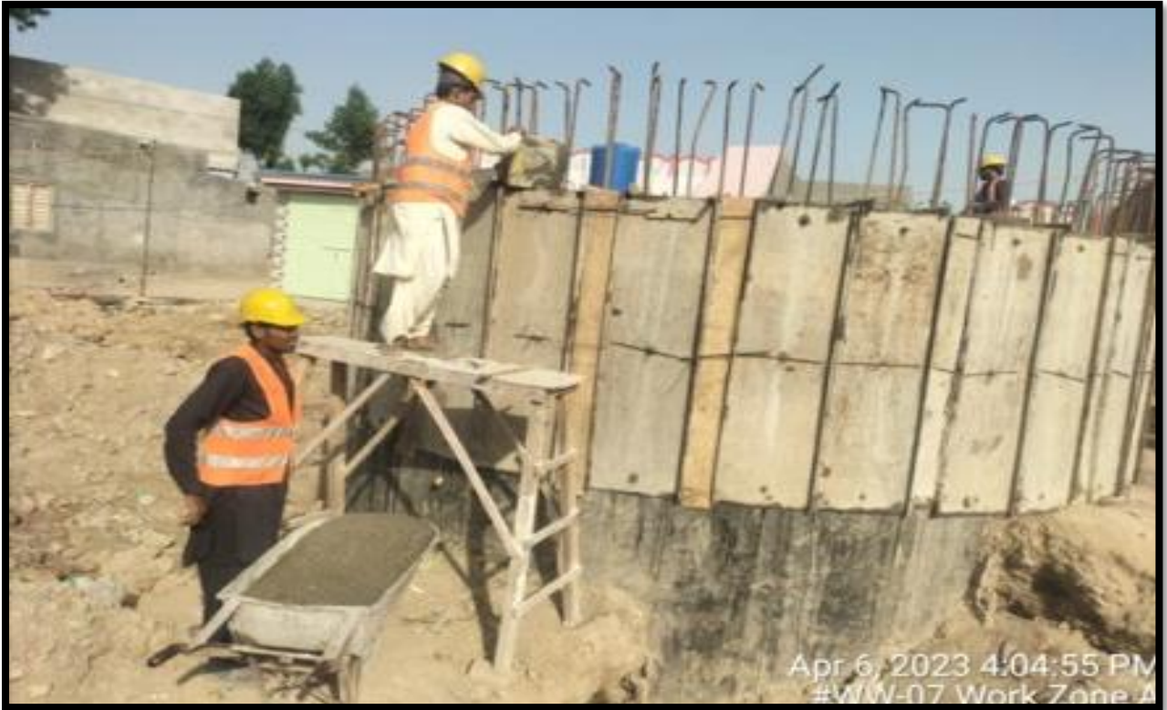
WW-07 (Zone-A) Concrete pouring of Sump at ADC colony work in progress
