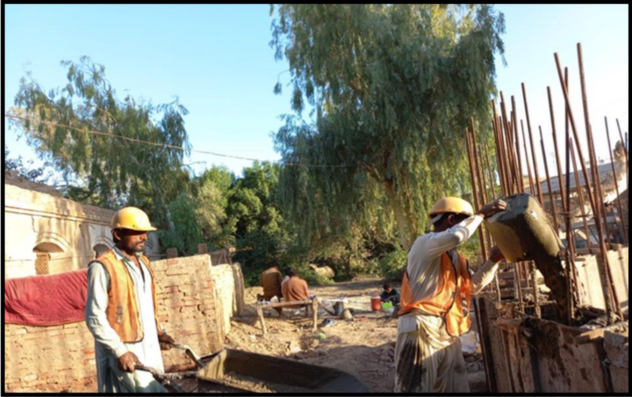
WW-09 (Zone C) Concrete pouring of Circular of Sump work is in progress
