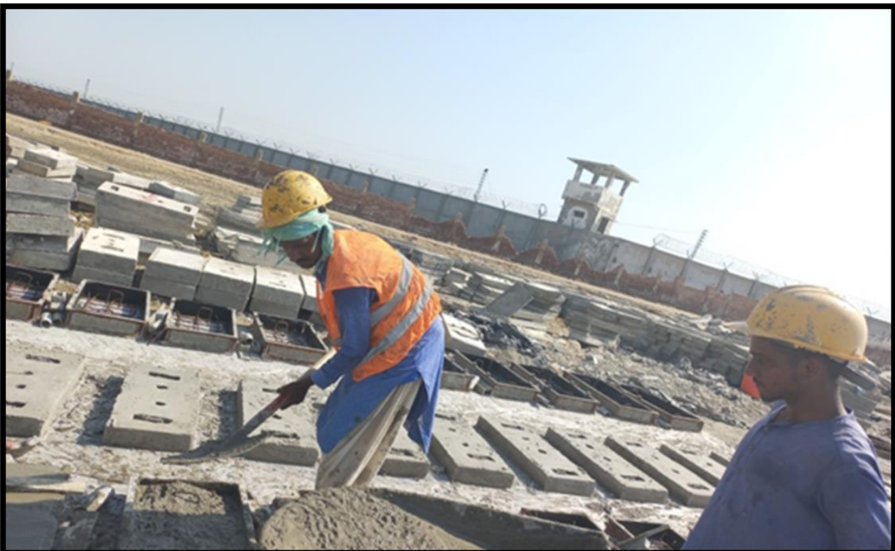
WW-07 (Zone-A) Concrete pouring of precast slab at Yard work is in Progress
