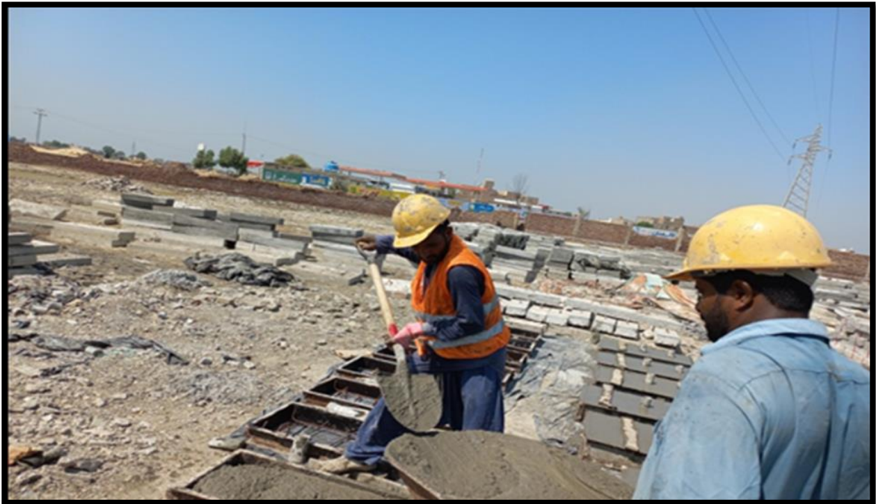
WW-07 (Zone-A) Concrete pouring of precast slab at yard work is in progress
