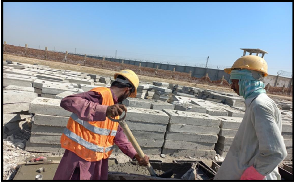
WW-07 (Zone-B) Concrete pouring of precast slab at Yard work is in progress
