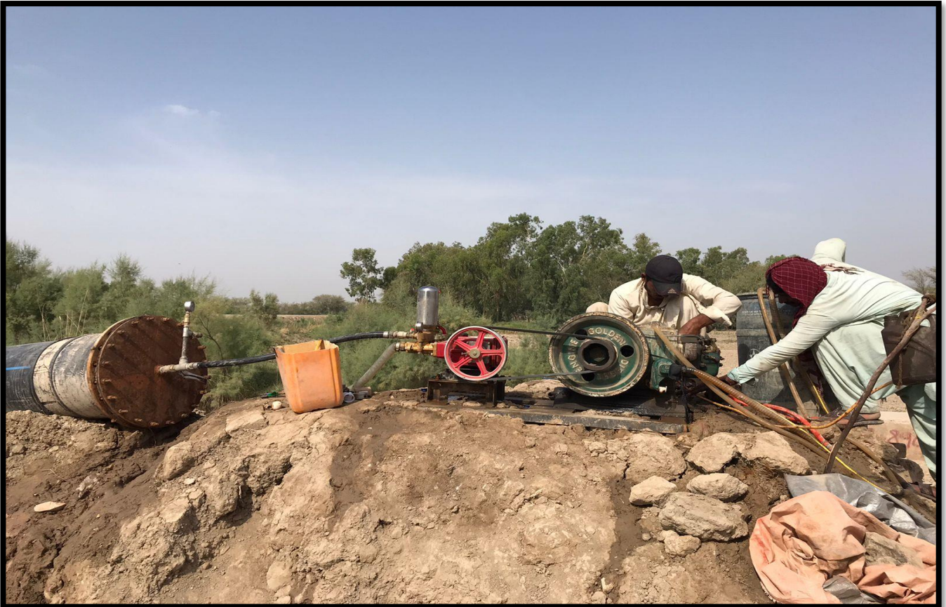
WW-12 (Zone-C) Filling of pipe for hydrostatic pressure test 500mm dia of Rising Main work in progress
