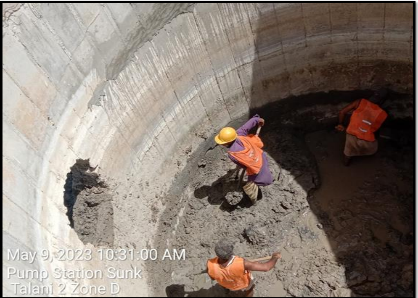
(Zone D) De-silting of Sump Talani-II for Sinking purpose work in progress
