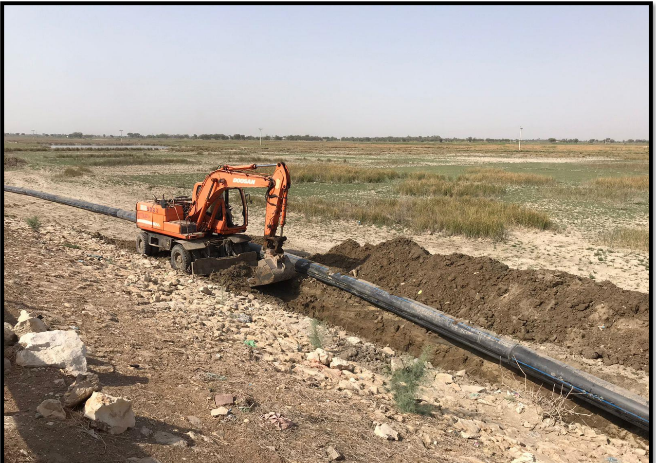
WW-12 (Zone-C) excavation for lying 500 mm dia pipe for Rising Main work in progress
