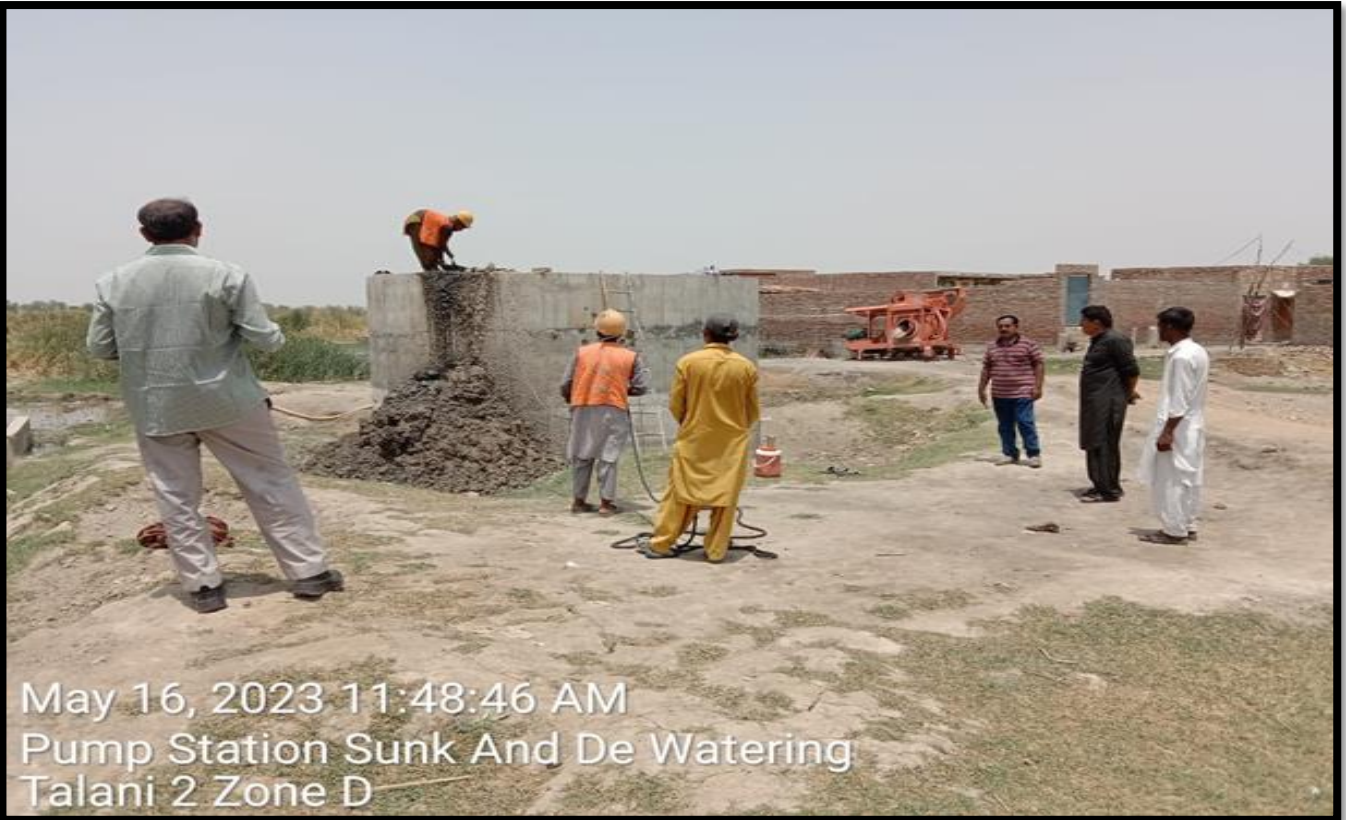
(Zone D) De-silting of Sump Talani-II for Sinking purpose work in progress
