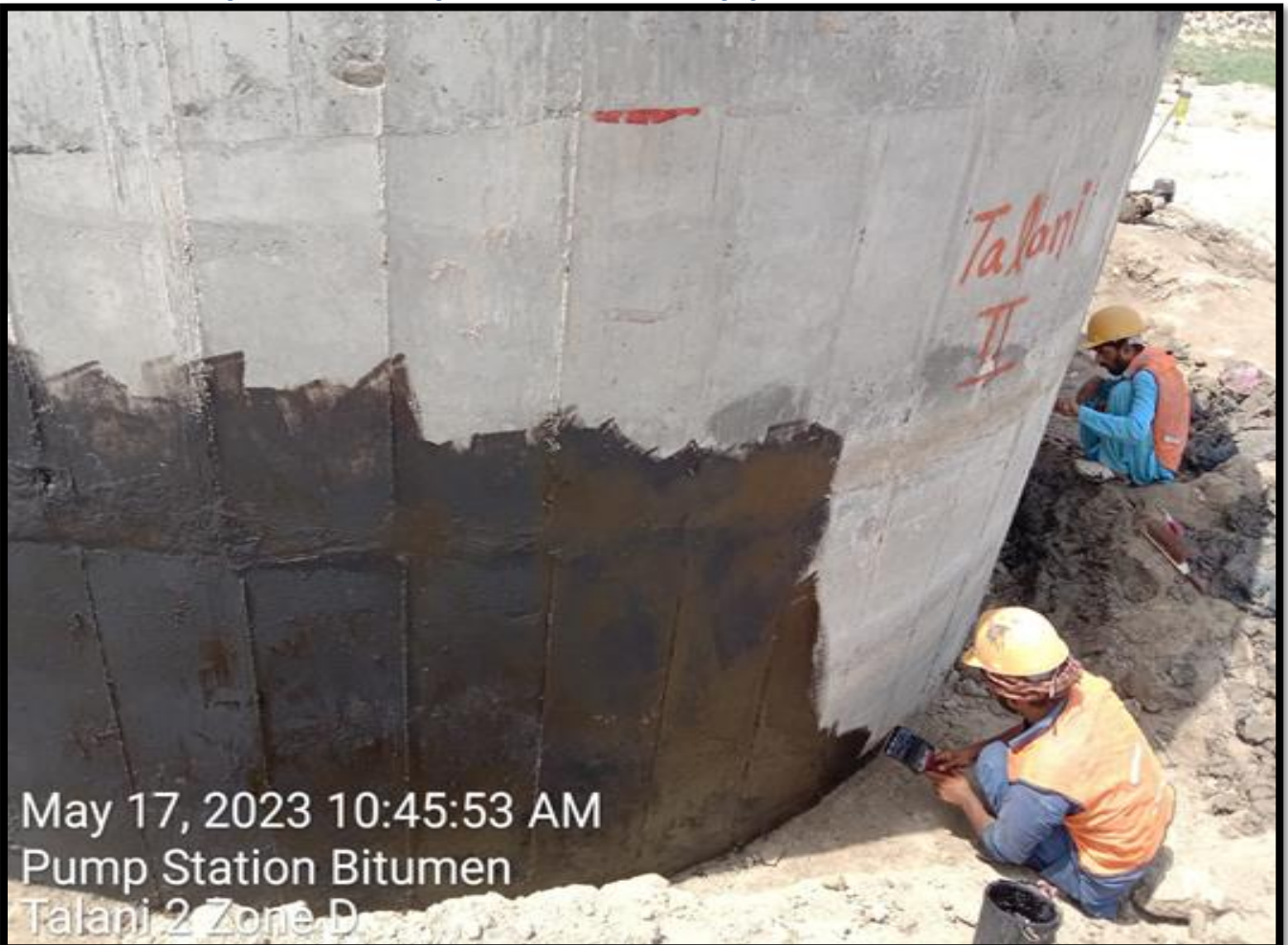
WW-10 (Zone D) Black Japan bitumen coat on Sump outside wall at Talani-II work in progress
