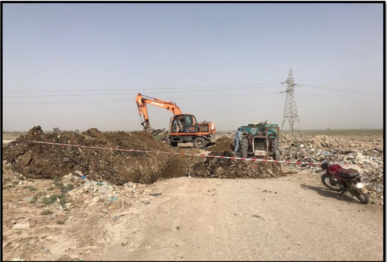
WW-12 (Zone-C) Excavation for laying 500mm diameter Rising Main work is in progress
