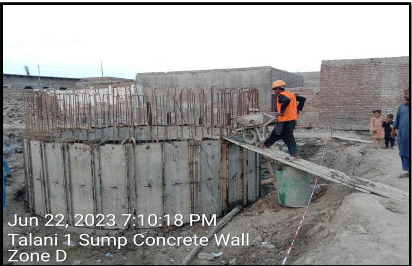
WW-10 (Zone D) Concrete pouring of Sump at Talani-I work is in progress
