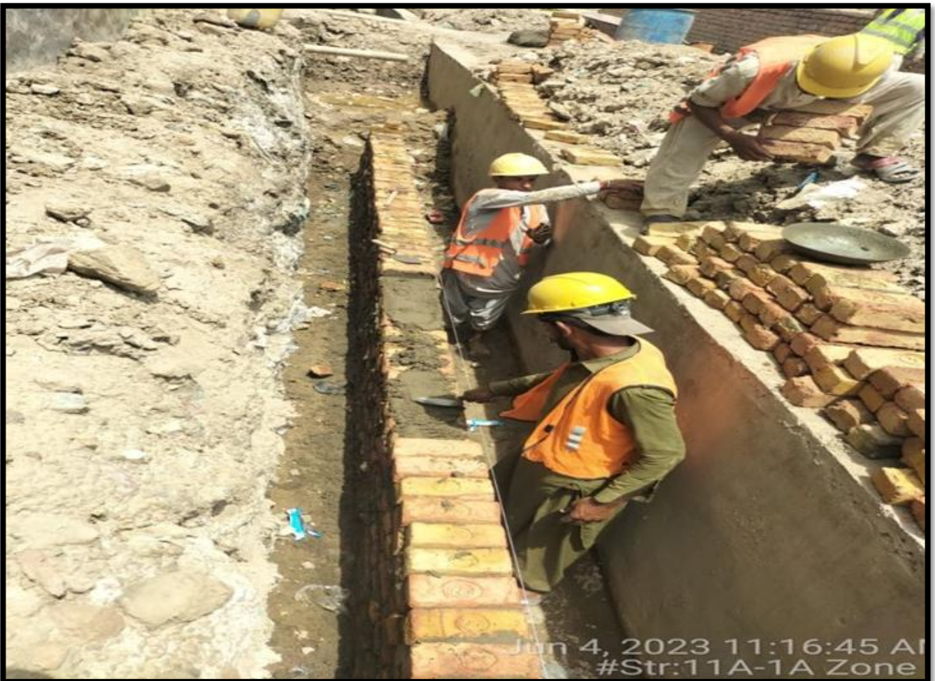
WW-08 (Zone-B) Brick Masonry of Drain Street No. 11 A1 at Al Murtaza Colony work is in progress
