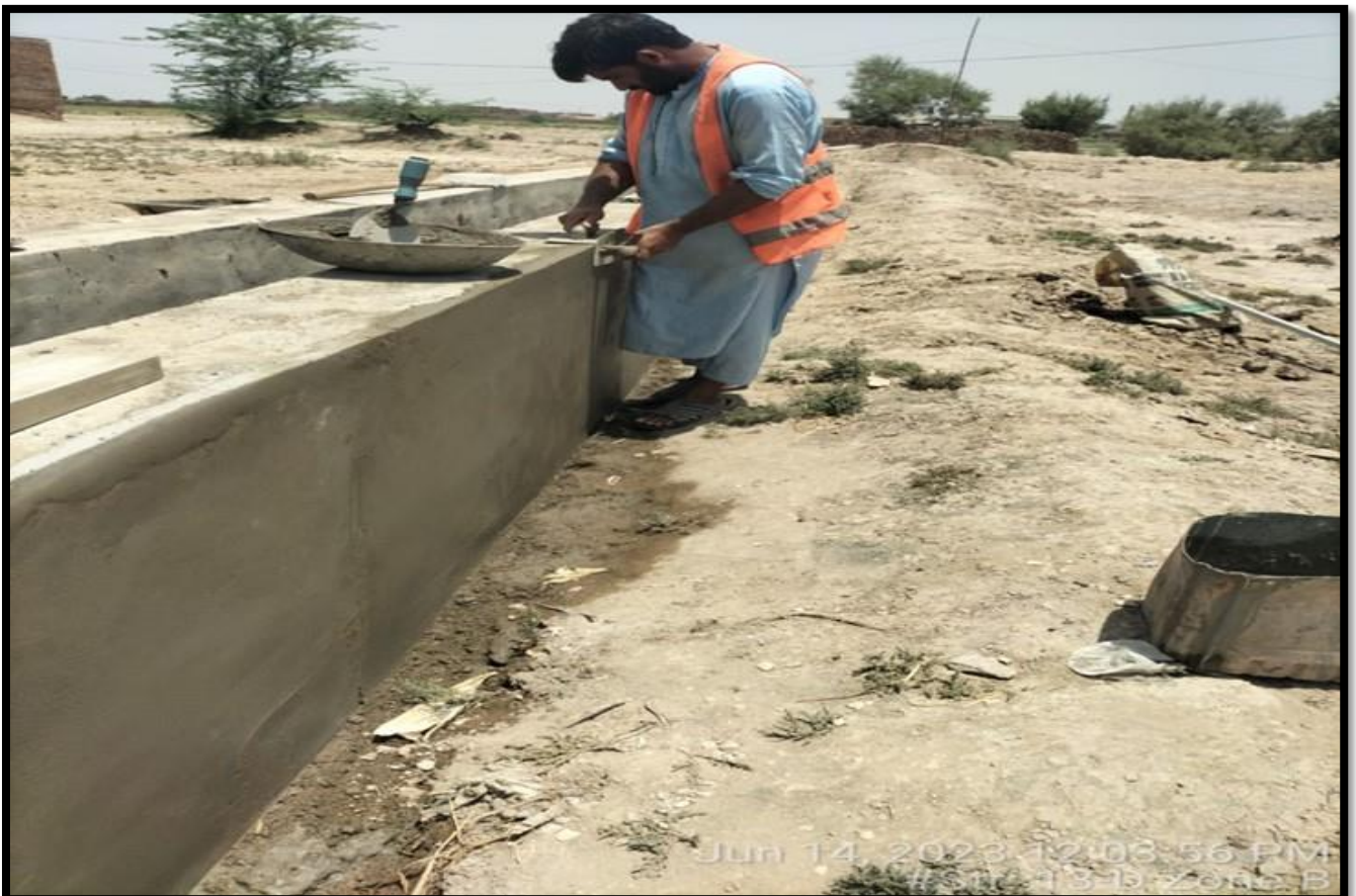
WW-08 (Zone-B) Curing of Brick Masonry drain Al Murtaza colony work is in progress
