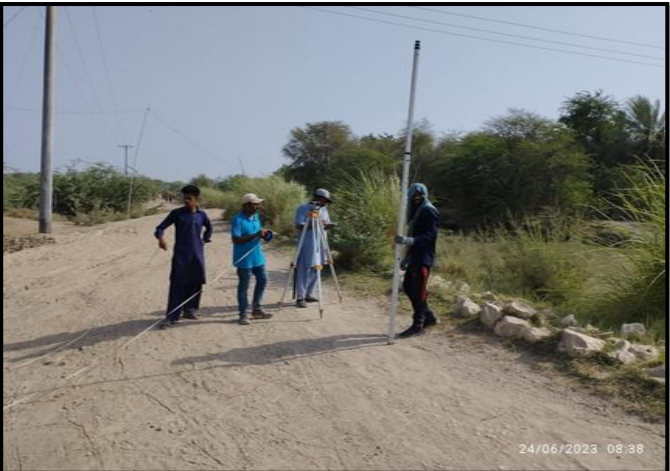
WW-19 During Survey of 500mm diameter Rising Main Aqilpur to Noor Wah work is in progress
