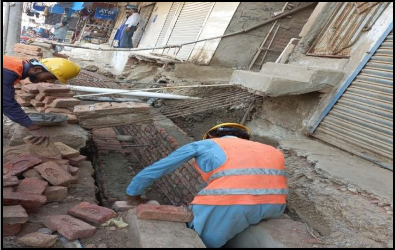
WW-08 (Zone-B) Brick masonry at street No. 67-A1 work is in progress
