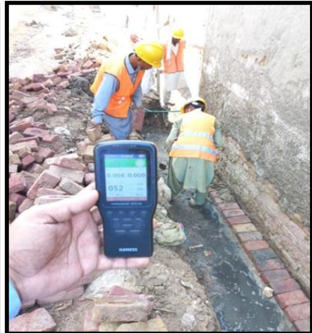
Monitoring of Air Pollution level with help of FORMALDEHYDE DETECTOR at site
