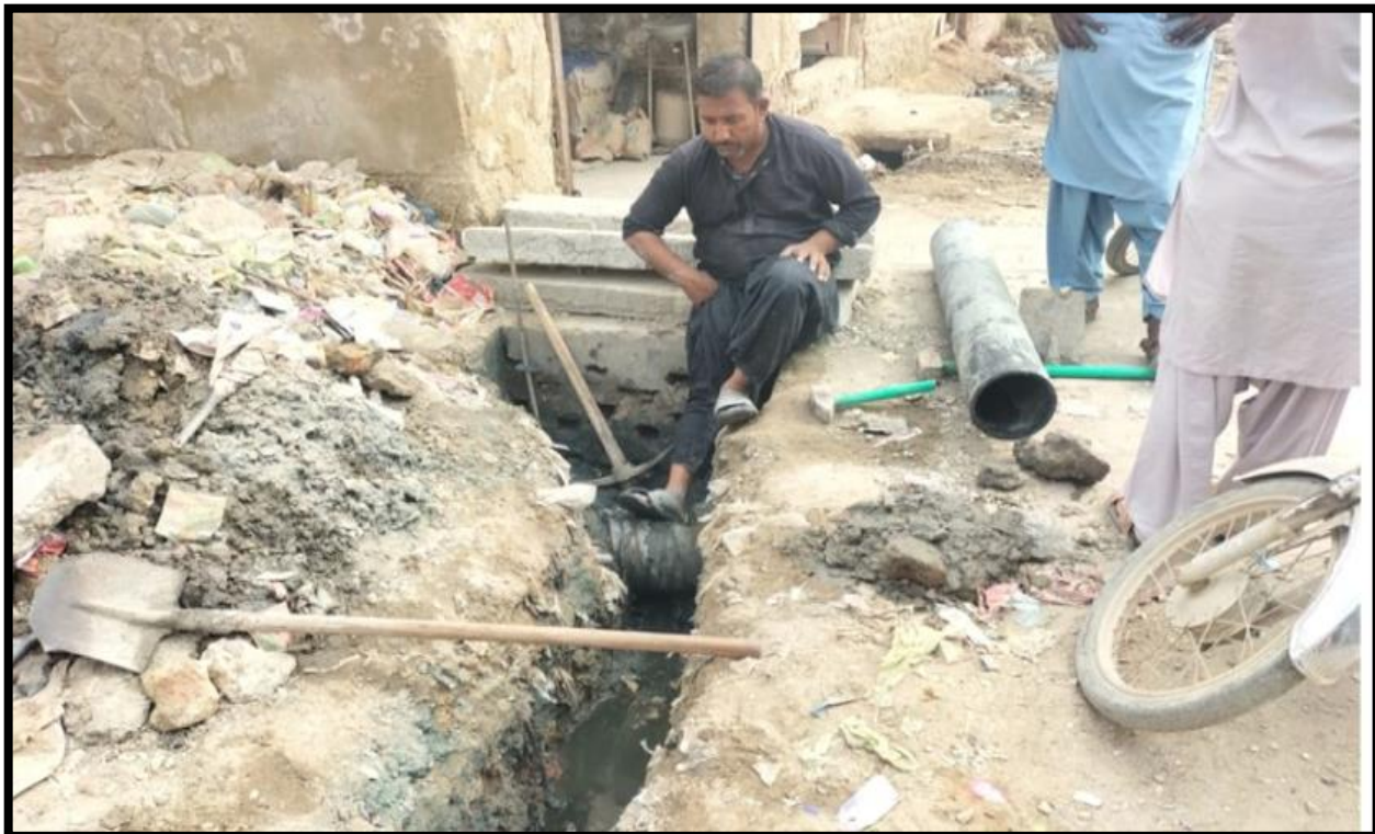
WW-07 (Zone-A) Excavation for pipe connection of Chamber with Bliss work is in Progress
