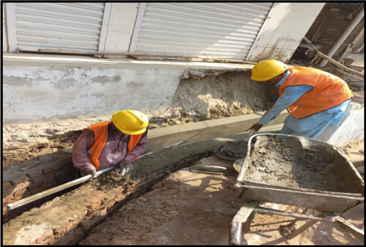
WW-08 (Zone-) Plaster of drain at street No. 67-A work is in progress
