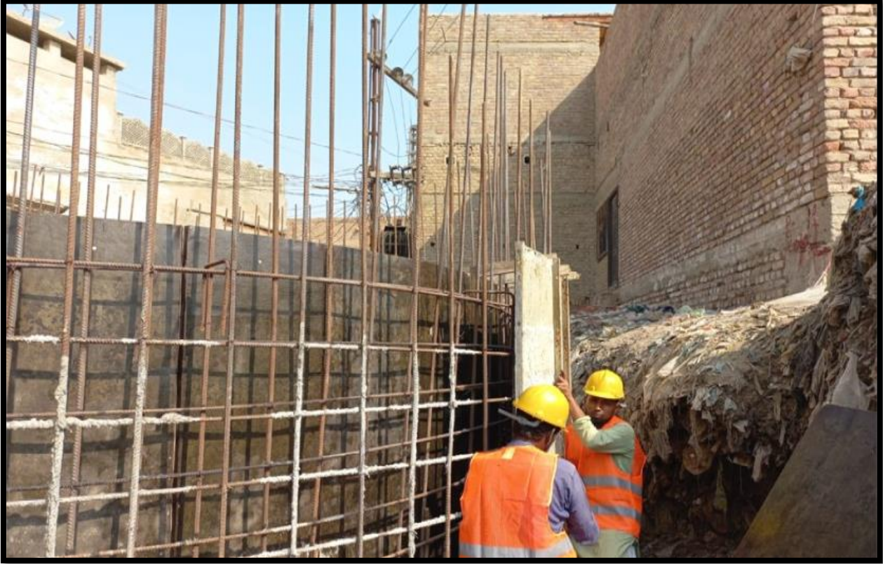
WW-07 (Zone-A) A concrete pouring for Phool Bagh work is in progress
