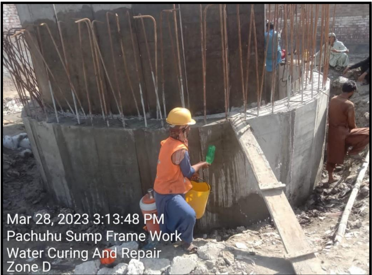
WW-10 (Zone-D): Formwork, water curing, and repair is in progress at Pachuhu Sump
