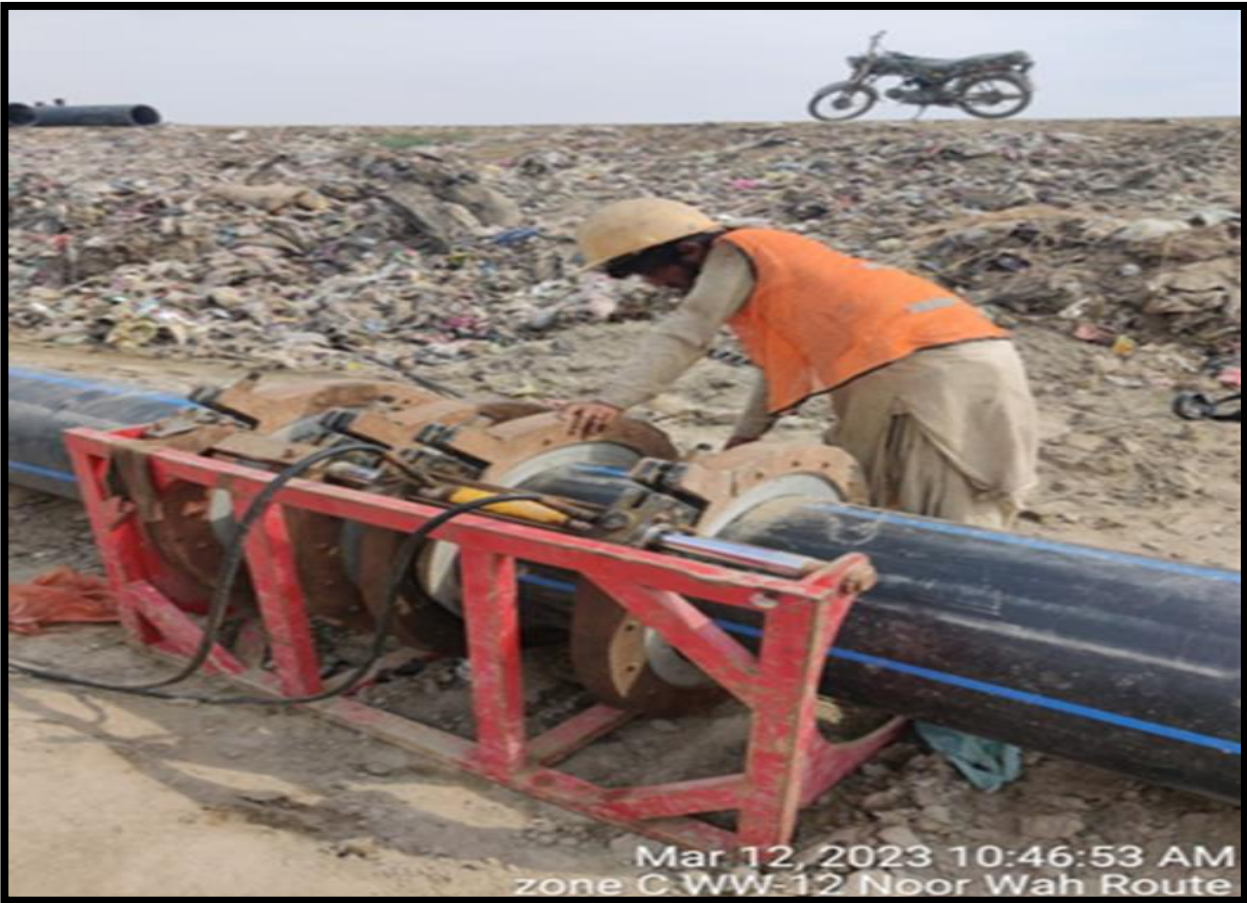
WW-12: Jointing of 500mm dia pipe for Rising main is in progress at Shamb-e-Shah to Noor Wah
