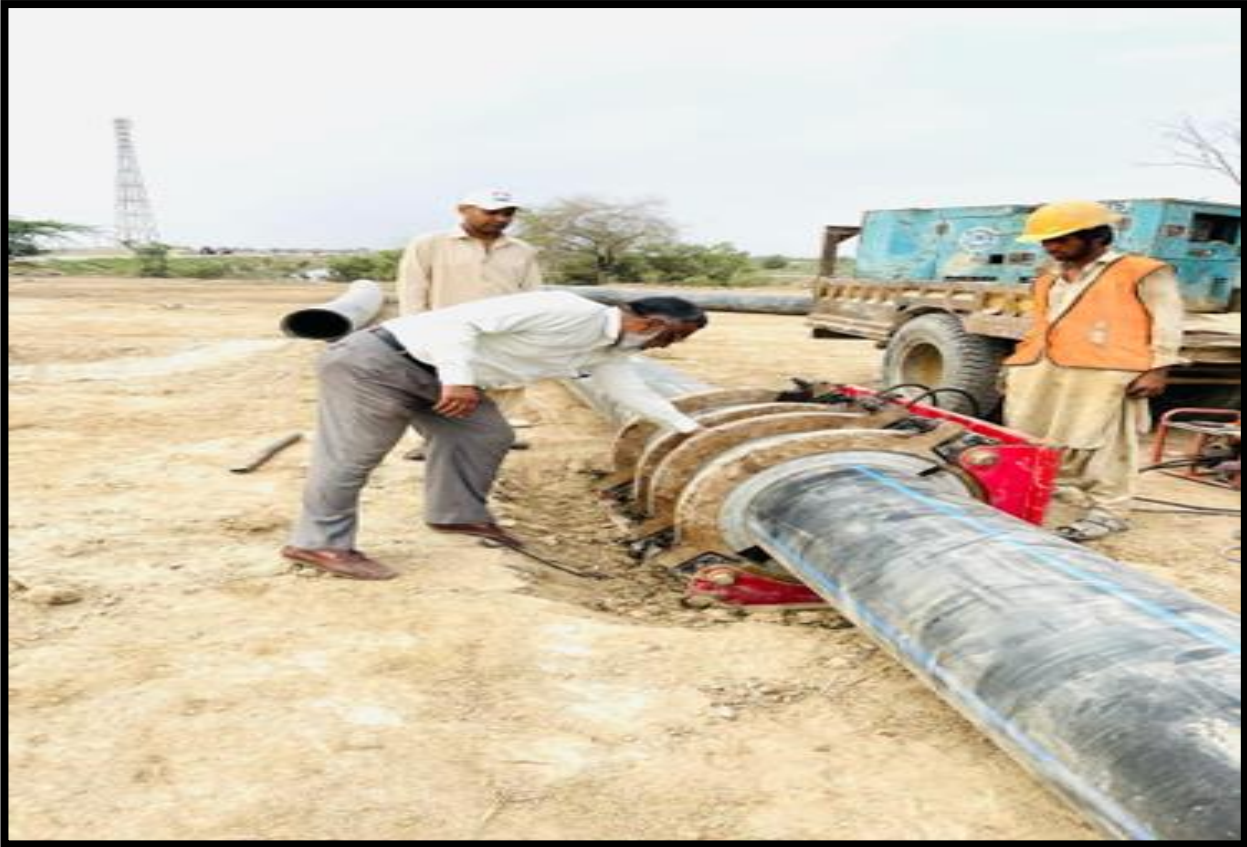
WW-12: Jointing of 500mm dia pipe for Rising main is in progress at Shamb-e-Shah to Noor Wah
