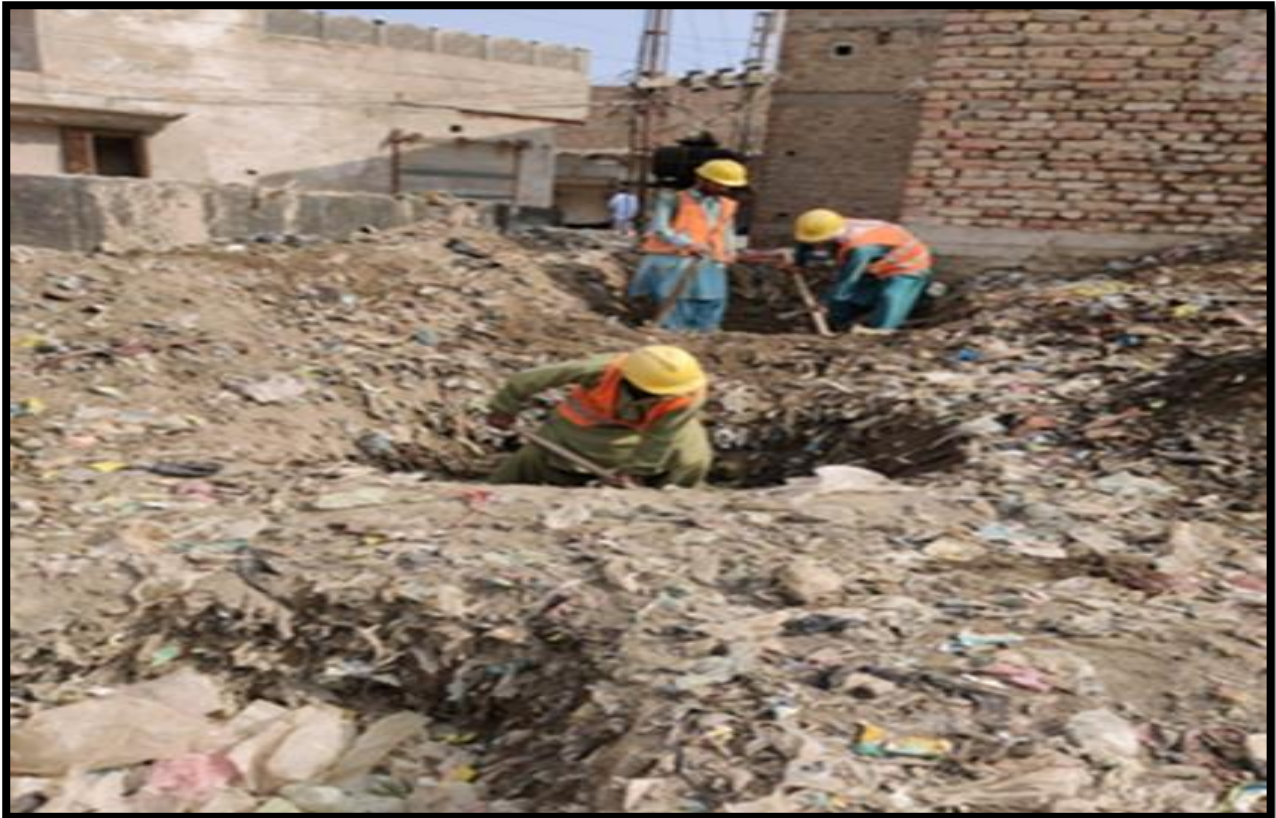
WW-07 (Zone-A): Excavation of footing for boundary wall of Phool Bagh disposal work in progress
