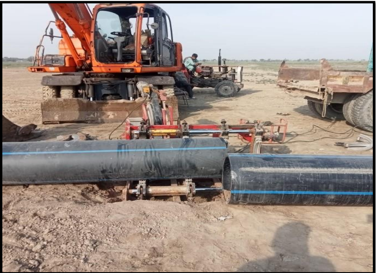
WW-12: Jointing of 500mm dia pipe for Rising main is in progress at Shamb-e-Shah to Noor Wah
